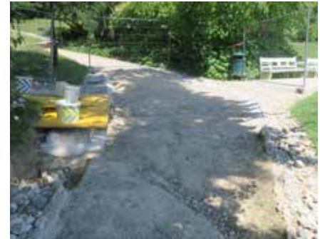
Fig. 98 The maintenance of the Kurgardens is never ending. Reconstruction works on the parkway sewage system in 2019.
